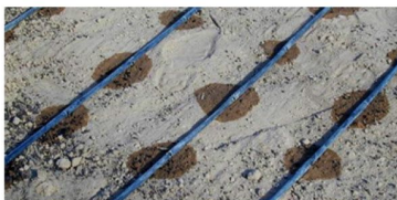
The above image shows the surface spread of moisture from the drip lines.
