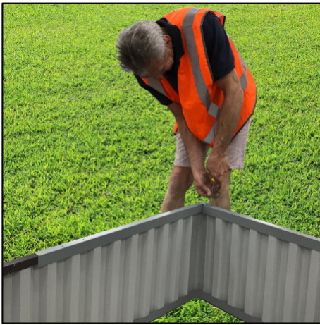
Figure 4. Securing the top rail to the wall panels, with the joiner insert in place.
